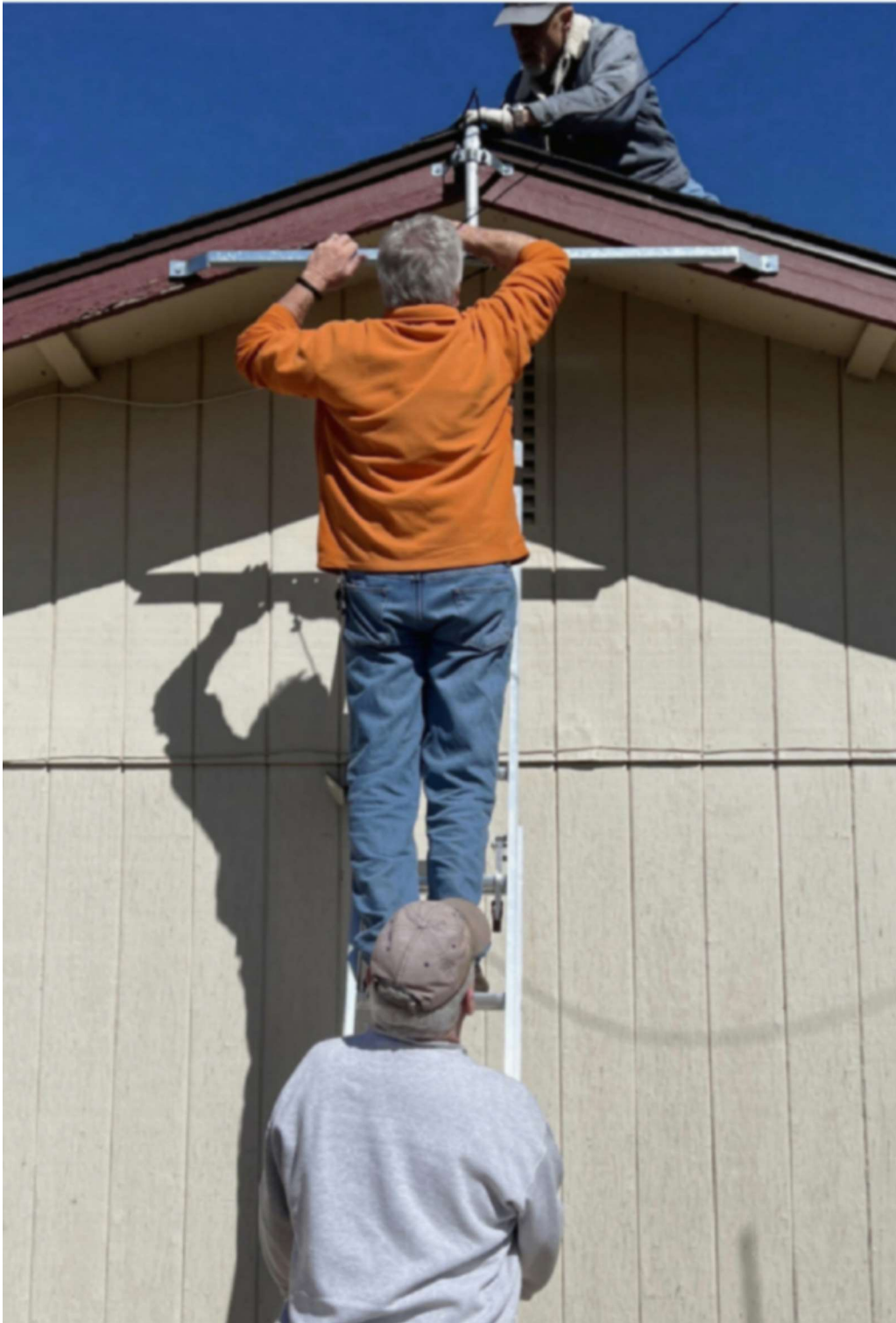
The YARC Elmer Crew (Top to Bottom: Art KG6AY, John KT7P, and Jim N6KZ) repairing an antenna after wind damage, February 24, 2023 (Photo courtesy of Raymond Kolman KI7COM).
